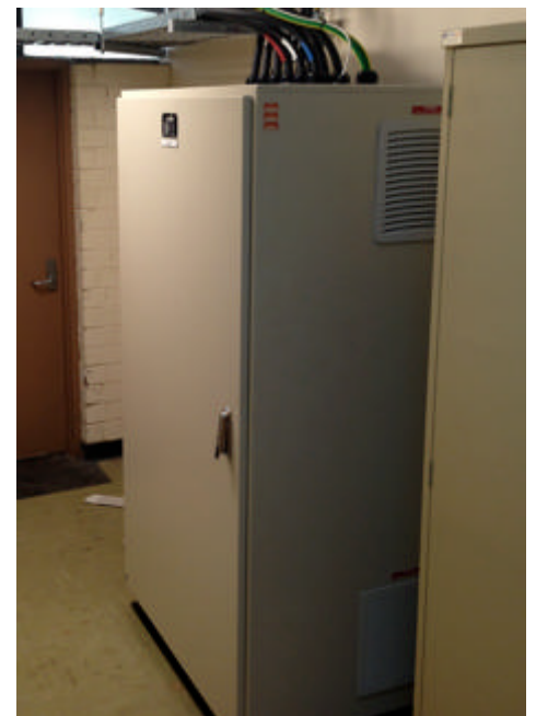
The Energy Saving unit was installed next to the site main switchboard. Incoming electricity is routed through the unit, and is refined and improved before it enters the buildings.
